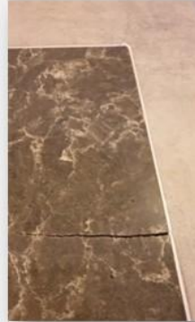
Typical Mechanical Crack Straight
